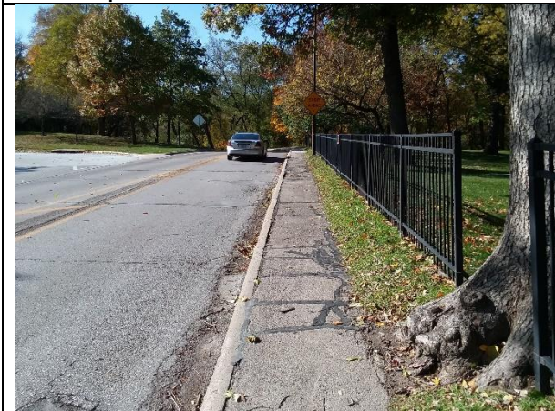
On Ontario Street the sidepath is very narrow and in poor condition.
